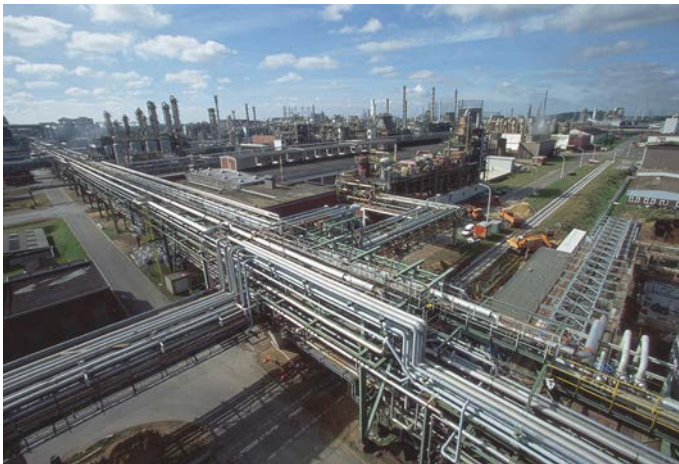
Figure 1-1 Pipes at Marl Chemical Park
